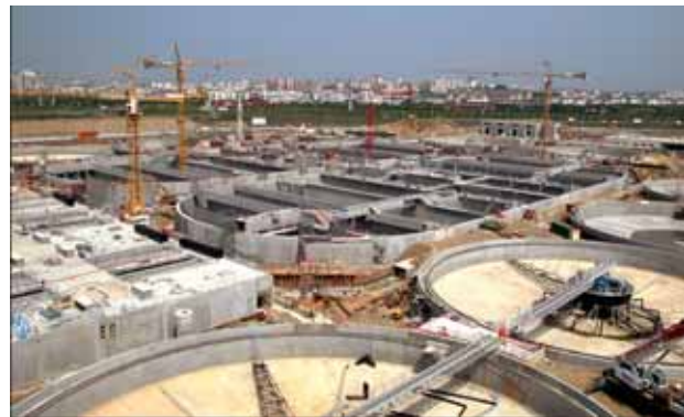
Seine amont treatment plant extension
